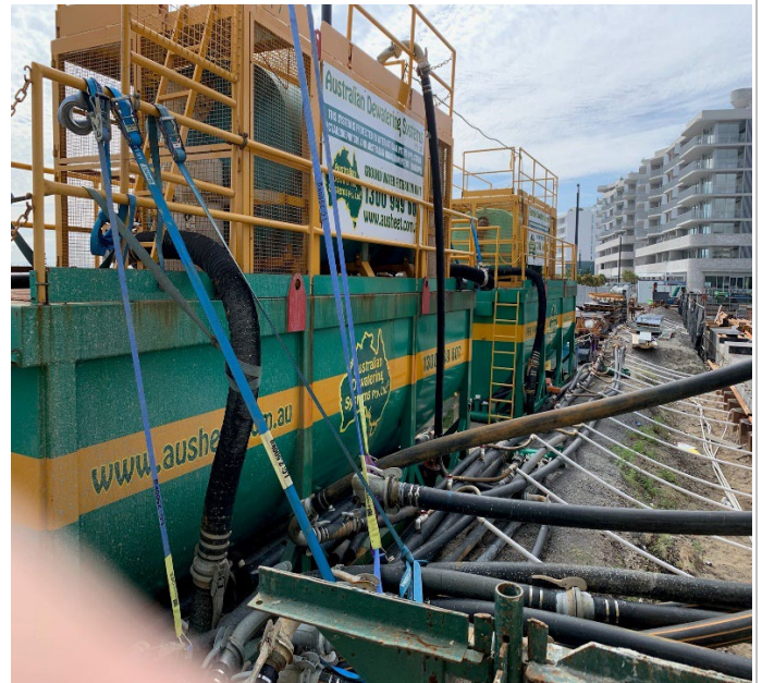
Photo 4: Groundwater Treatment unit
